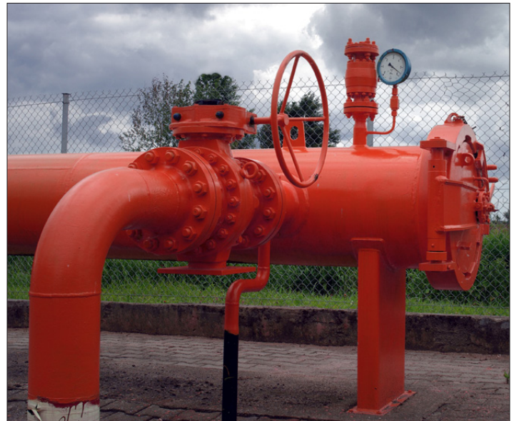
Barrel Style Pigging System
